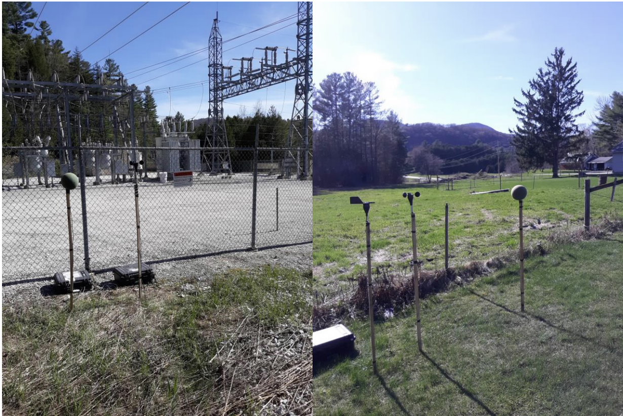
FIGURE 9: PHOTOGRAPHS OF THE SUBSTATION MONITOR (LEFT) & RESIDENCE MONITOR (RIGHT)
