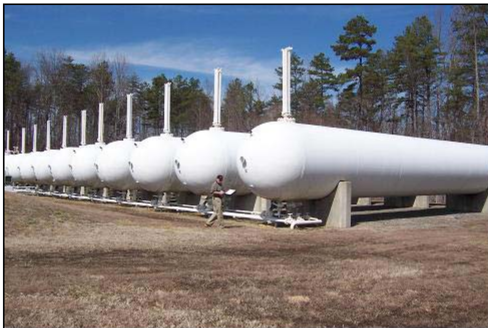
Figure 2 Propane Storage Tank Facility
