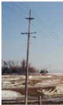
46 kV transmission lines Location unknown Credit: CVPS
