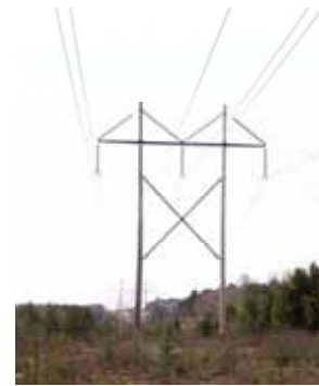
345 kV transmission line Coolidge area, VT Credit: VELCO
