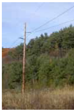
115 kV transmission line West Rutland, VT Credit: VELCO
