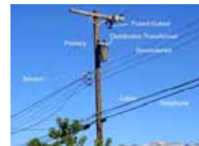
Distribution Pole with transformer and telephone lines Credit: US DOL
