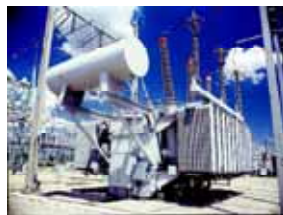
Distribution Substation Transformer Credit: US DOL
