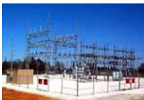
Distribution Substation Credit: US DOL
