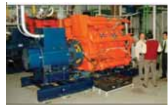
0.8 MW reciprocating engine Credit: DOE
