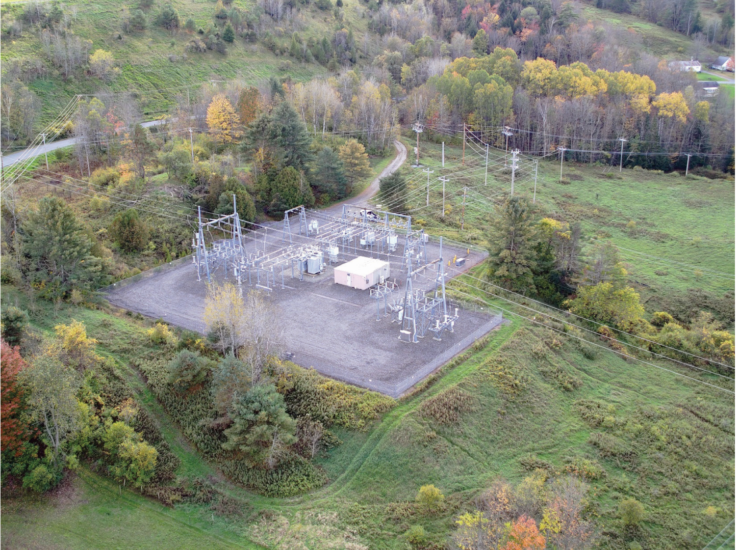
Figure 3: Oblique aerial view of the existing substation and surrounding overhead transmission and distribution facilities. This view is looking roughly south from the north, with Higgins Hill Road visible in the upper left side of the image.
