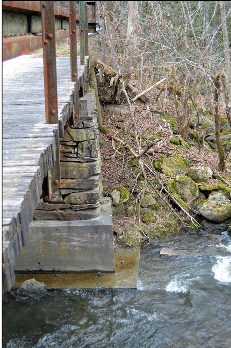
PLATE 63: South Abutment of Pony Truss Bridge, Falls Road over Mill River, Georgia, Looking Southwest
