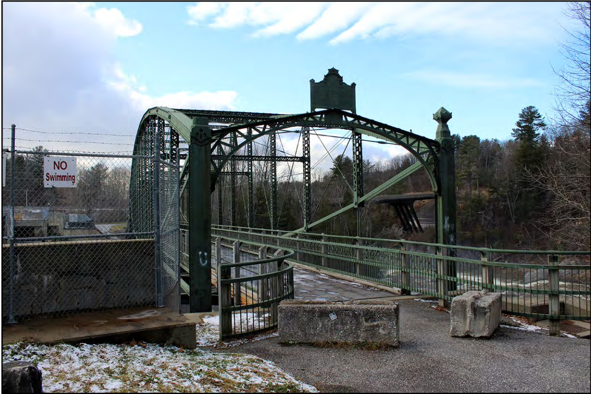
PLATE 6: Douglas & Jarvis Patent Parabolic Truss Iron Bridge, Crossing the Missisquoi River, Looking West
